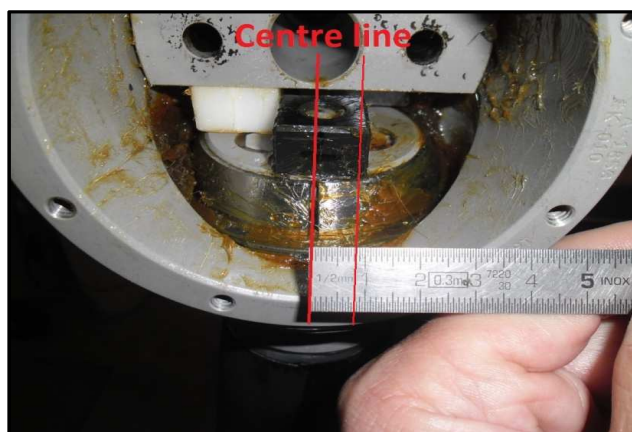
Fig. 8: Correct ! Split line is min 8 mm (0,314 inch) from the pitch damage pin!
