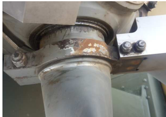
Figure 2: Corrosion on counterweight body and screws
