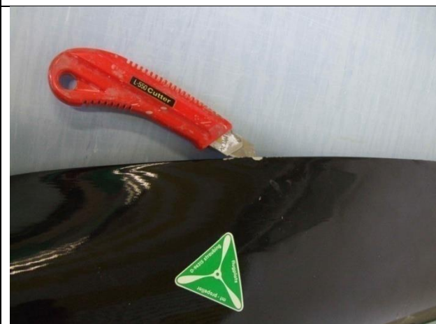
Delaminated composite shell on the trailing edge
